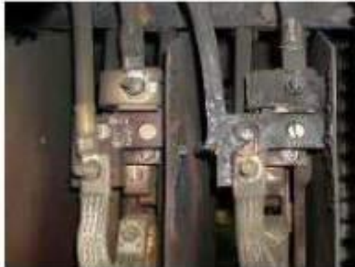
▲ Due to condensation, the circuit breaker has failed
